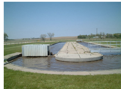
Laurel wastewater treatment plant oxidation ditch.
